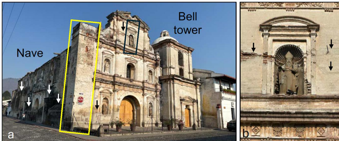
Figure 10: Oblique view of the front (east) façade and south wall of the Church of San Agustín and bell tower showing antiseismic structural elements and earthquake damage. a) The white arrows point to exterior buttress walls at the base of the south wall of the church. The yellow box outlines the southeast structural corner tower. b) Statue of San Agustín holding a church located in the upper central niche of the church façade. Note the horizontal cracks marked with arrows that cross laterally through the niche and bifurcate into cracks on the north side, demonstrating clear earthquake damage.
