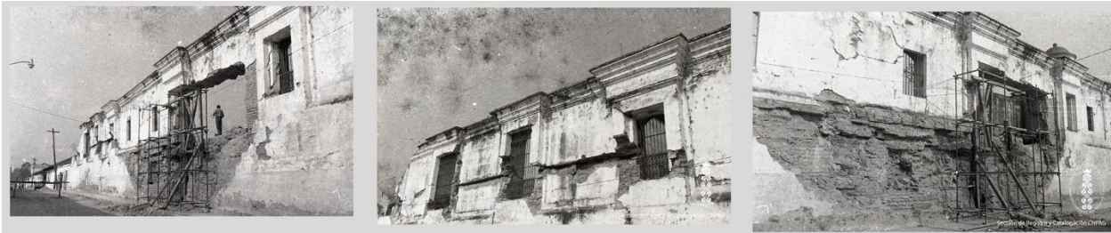
Figure 6: East wall of the Palace of the Captains General showing collapse and shearing of the exterior east wall (Photos courtesy of CNPAG Sección de Registro y Catalogación).
