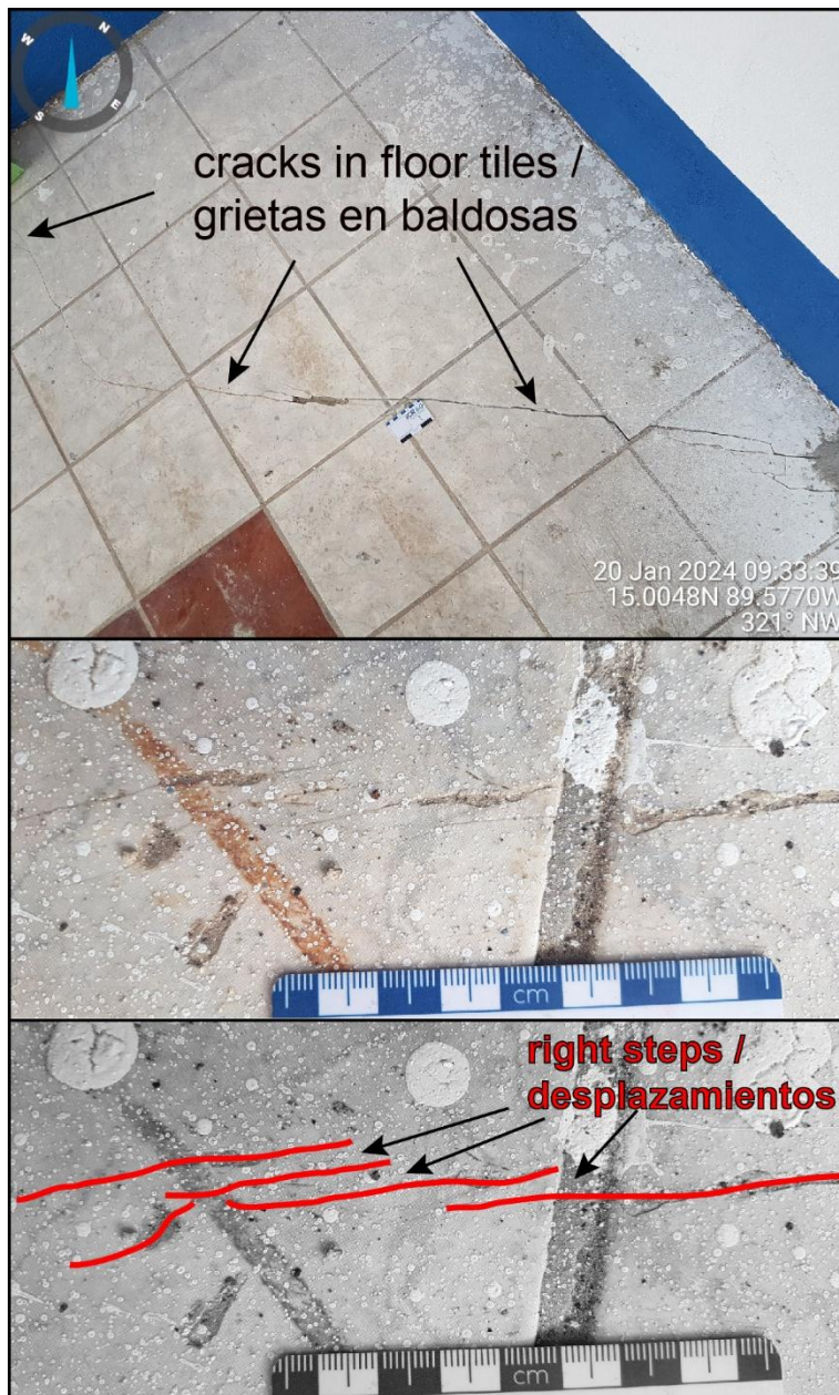
Figure 18: Cracked floor tiles show right-stepping en-echelon geometry and millimeter-scale offsets.
