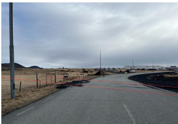
Figure 2: Field photograph showing the resistivity system survey crossing surface fractures in central Grindavik in 2024.
