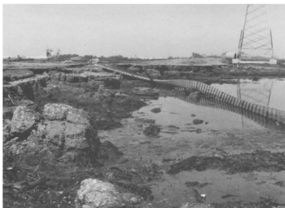
Figure 6: Heavily deformed railway tracks in the area flooded by the tsunami in Lázaro Cárdenas. (Photo taken from Lomnitz and Castaños, 1985). | ESI-07 = X.
