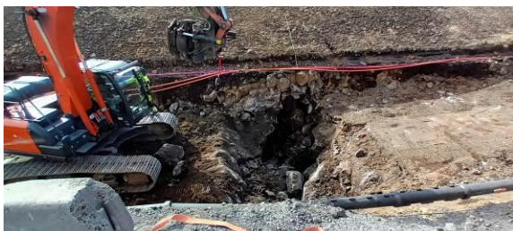
Figure 5: Field photograph by G. De Pascale showing a subsurface horizontally open fissure in bedrock as shown in the locations near station 150 on the horizontal axis in Figure 9 and 10. Please note that during the fixing of the road here, it provided an important opportunity for subsurface insight here as well as validation of the nature of the high resistivity values which in this instance are due to an open fissure at about 2 m below road level. Please note that the photo was taken at road level and the excavator was digging down to fix infrastructure in the subsurface and mitigate the fractures here (aka fill them in so that they did not collapse during future earthquakes). Please note that the zone at station 155 m was excavated and there was an open bedrock fissure there that was field validated coincident with the red coloured – high resistivity area below ~2 m depth.
