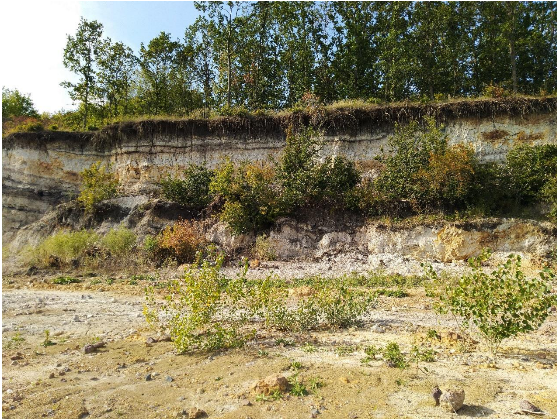
Fig. 17: Nechanice dam: Back-tilted blocks of old slumps with conserved vegetation.
