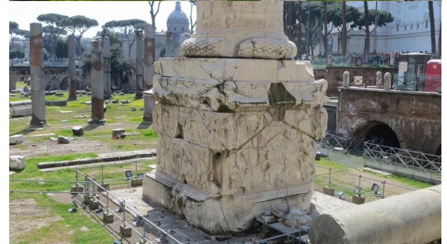
Fig. 2.4.3 – Above: Basilica Ulpia with the Column of Traianus in the background. Below: basement of the column with crisscrossing fractures, possibly due to seismic shaking
